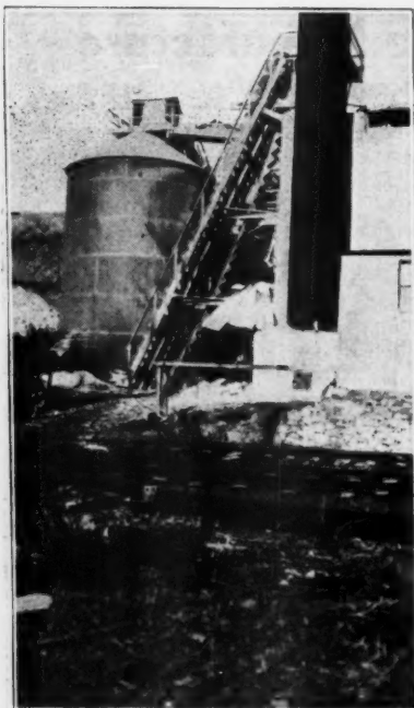
Crushed Stone Storage With Bucket Elevator to Rotary Kiln.
